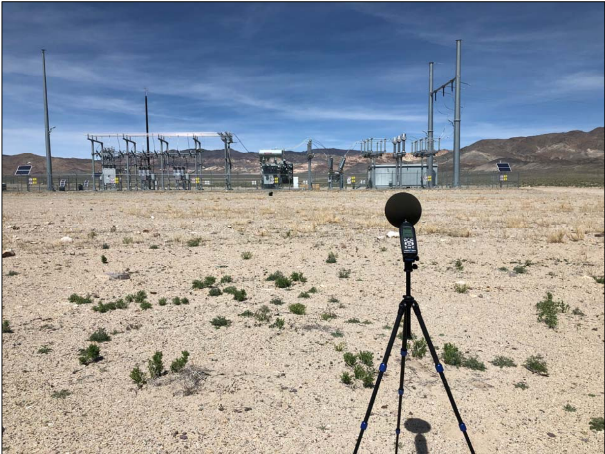
Figure 2-3. Photograph of the Table Mountain Substation
