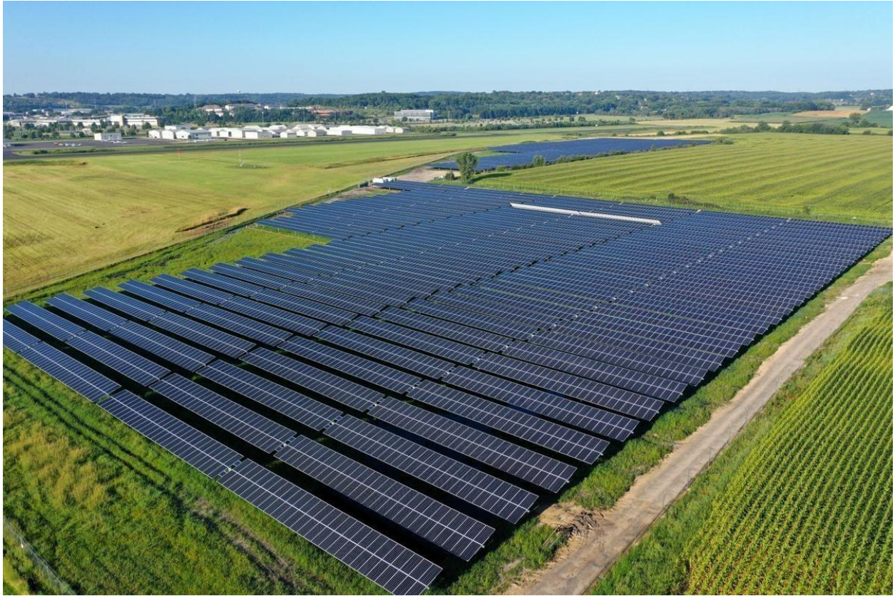
Figure 9 – Morey Field Solar Array next to Middleton Municipal Airport (Image source oneenergyrenewables.com )
