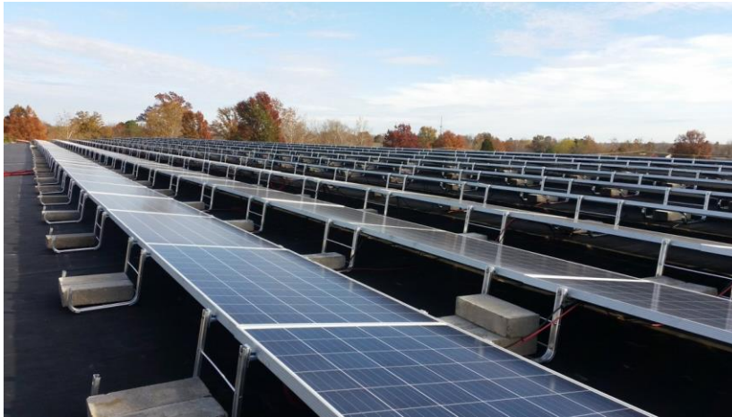
Figure 6 – Roof mounted solar at a 10-degree tilt
