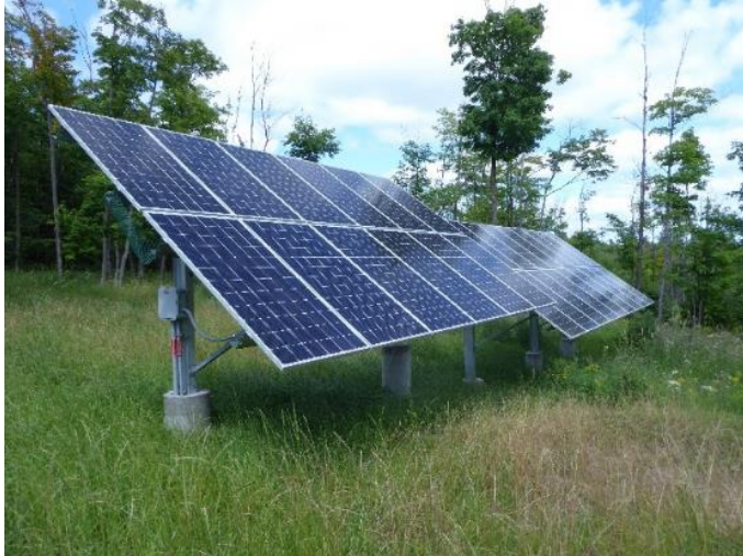
Figure 8 – Ground mount solar PV
