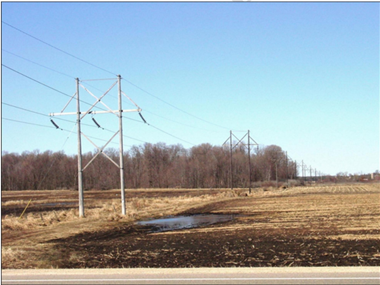
Figure 4-2 Typical two-pole H-frame structures (image is for illustration purposes only – structures are not necessarily those proposed for this project)
