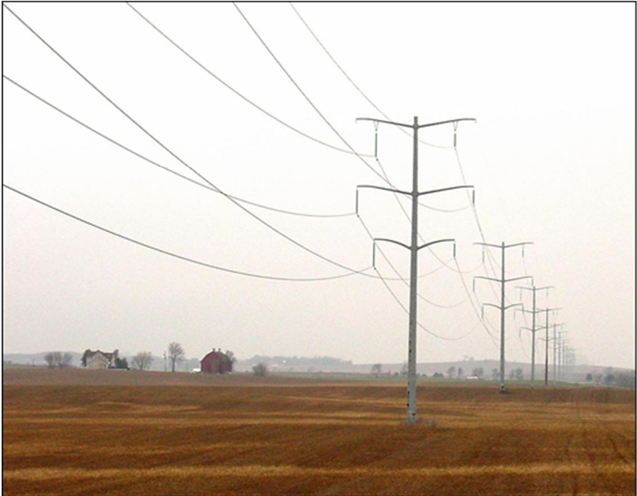
Figure 4-3 Typical single-pole double circuit structures (image is for illustration purposes only – structures are not necessarily those proposed for this project)
